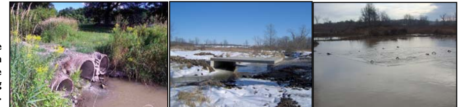
Fish Barrier #109 (left), the newly installed clear span bridge (middle), and the site submerged during the spring of 2007 (right).
